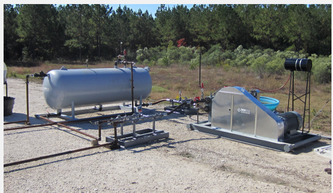
Tech-Flo's permanent installation after production testing with a natural gas unit.
