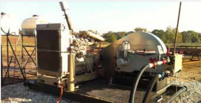
Tech-Flo's permanent unit with Cummins natural gas engine.
